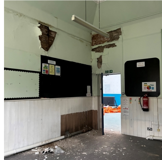
Classroom with crumbling lathe plaster walls
